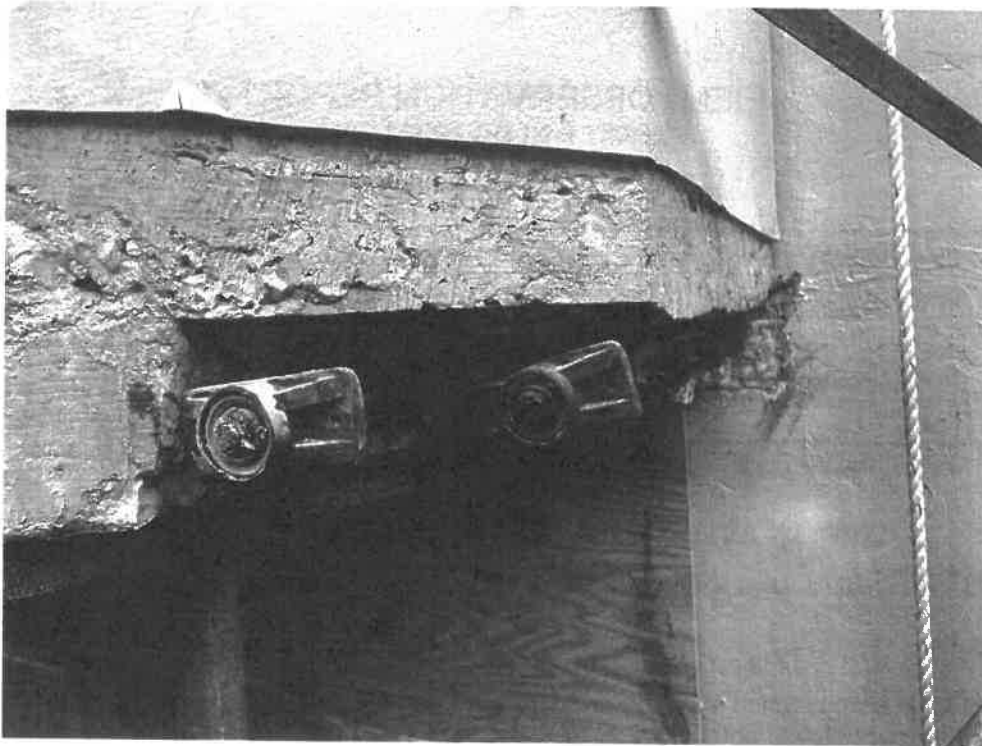
Photograph #1: In-progress post tension concrete repair at the balcony of Unit 2B5
