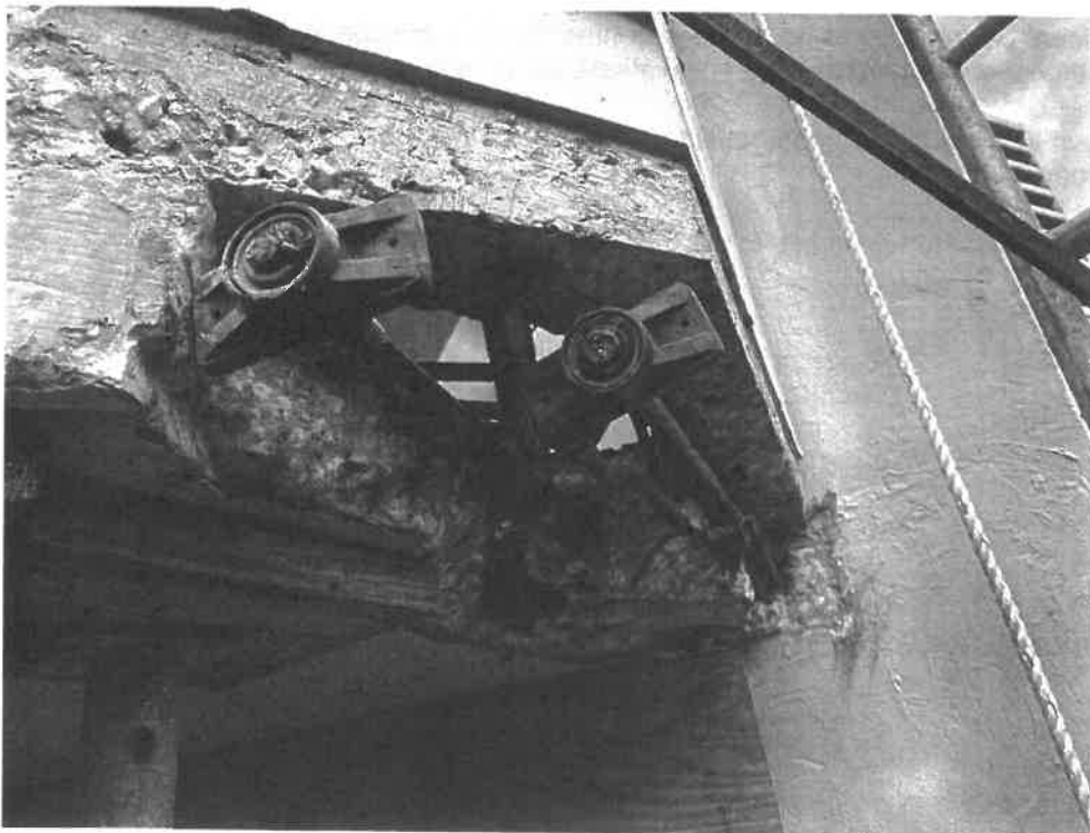
Photograph #2: In-progress post tension concrete repair at the balcony of Unit 2B5
