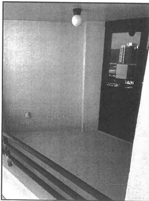
Photograph #2: Damage identified at the balcony of Unit 21A3
