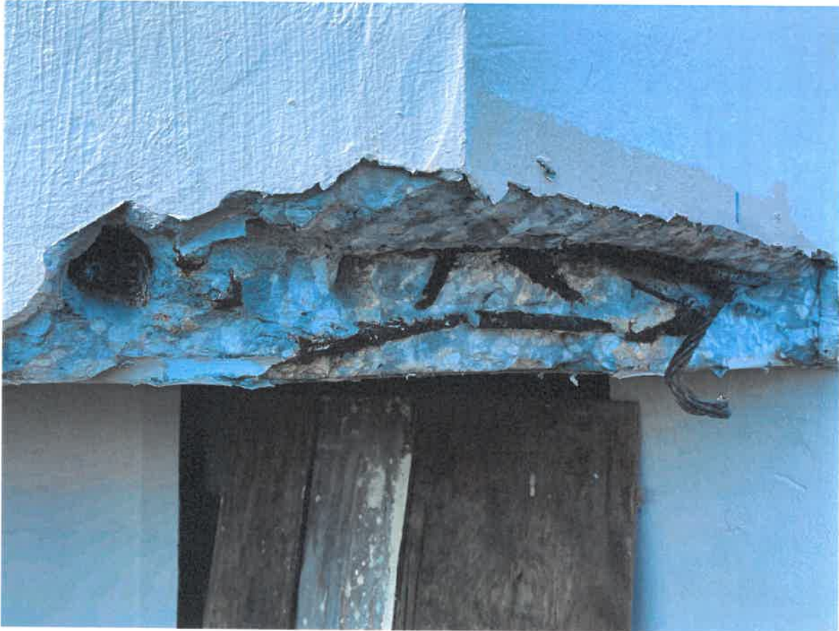
Photograph #1: Exposed broken post tension cable at Unit 2B5 balcony
