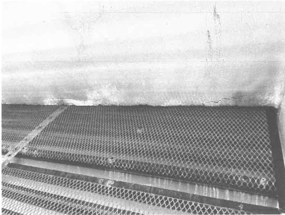
Photograph #3: Ceiling slab edge damage
