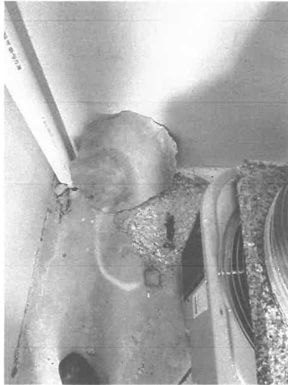
Photograph #1: Topside damage requiring A/C to be re-located
