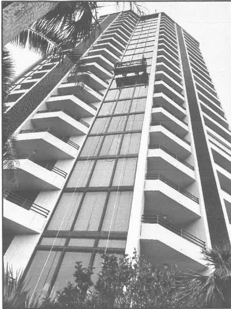
Photograph #1: Completed scope of work at the 06 window stack at Tower B
