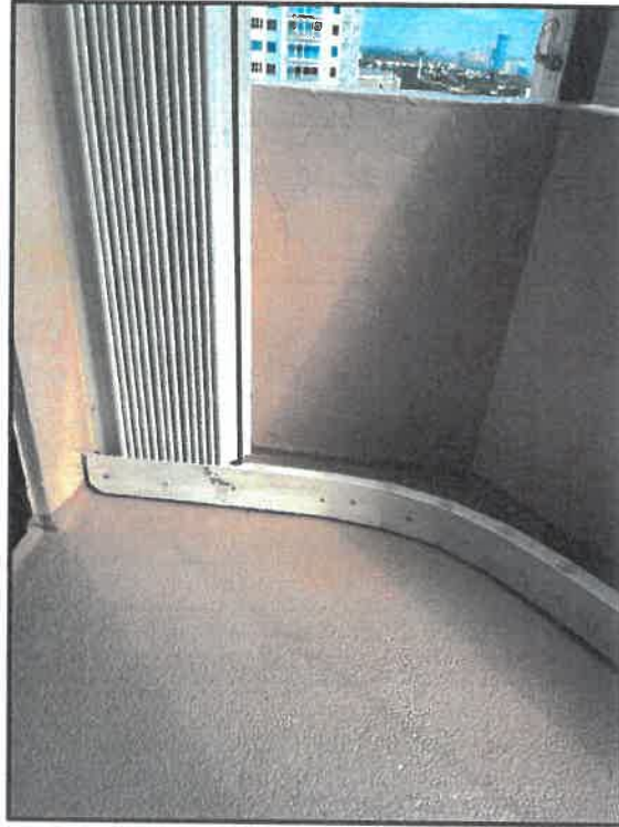
Photograph #1: Excess deck coating observed on the shutter track at the balcony of Unit 1702
